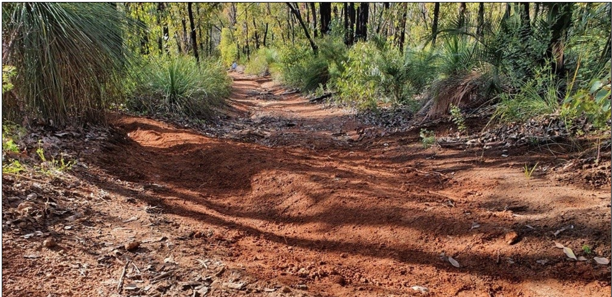
The reddish mound in the center of the photo is a covered water bar. The stones underneath lend strength and durability to the structure, while the mounded soil allows wheels to pass over. While this example is intended for mountain bikes, particularly firm and stable mounds may be able to meet FSTAG standards. Photo Credit: Bibbulmun Track ( bibbulmuntrack.org.au ).
