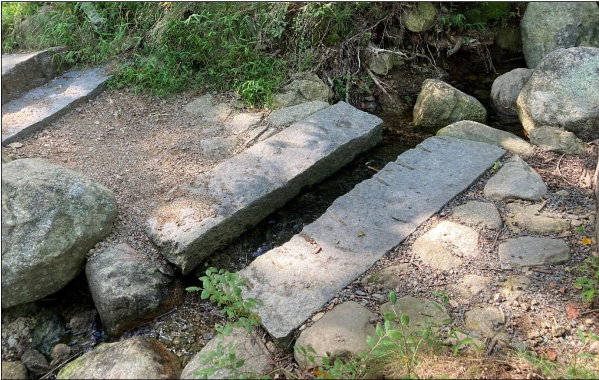
Open culvert using imported stone slabs. Always fails to meet FSTAG standards.
