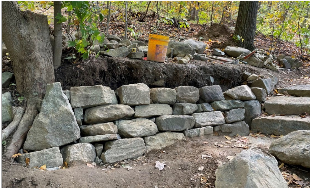
This retaining wall is built above the trail, to keep soil from sliding down onto it.
