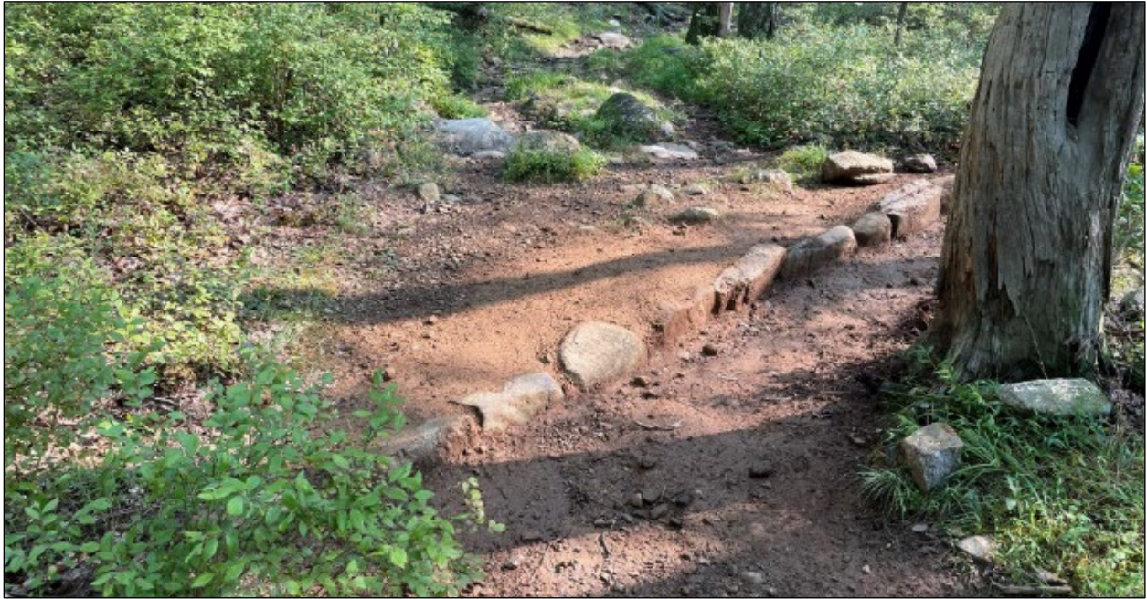
A classic stone waterbar. In this example, water would flow from the viewer toward the structure and then be directed off to the right of the trail.
