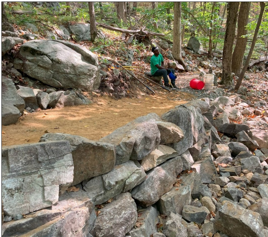
This crib wall is built below the trail, to allow a level and stable tread surface.
