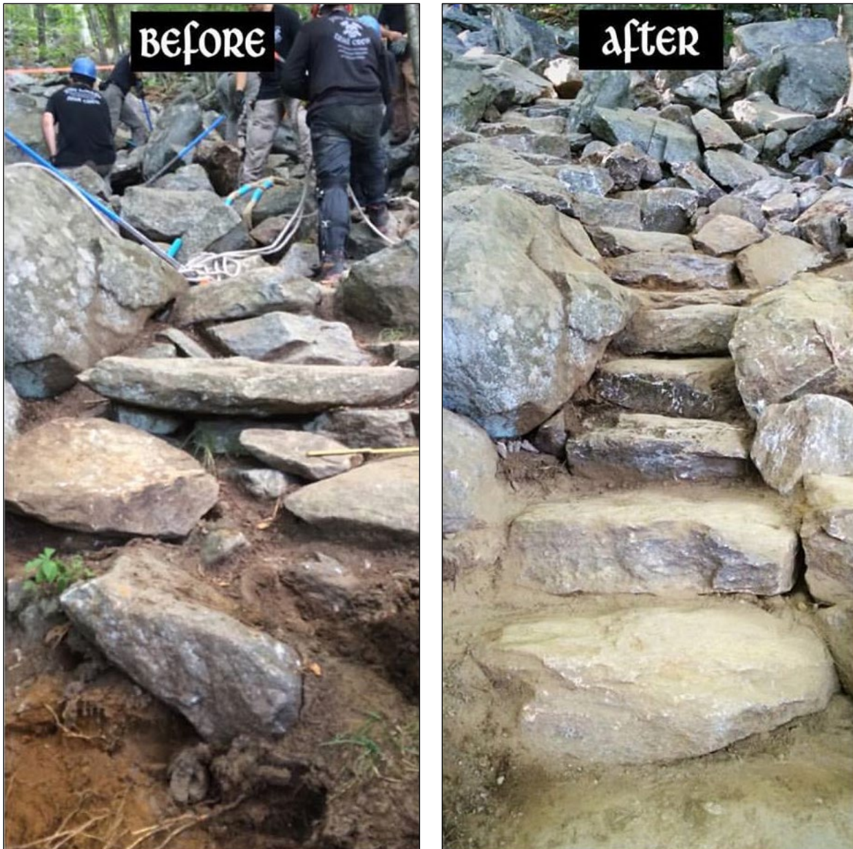
Before and after shots of a previously unsafe trail stretch converted to level, stable, and (relatively) evenly-spaced steps along a stone staircase. Photo Credit: Jolly Rovers Trail Crew ( jollyrovers.org ).
