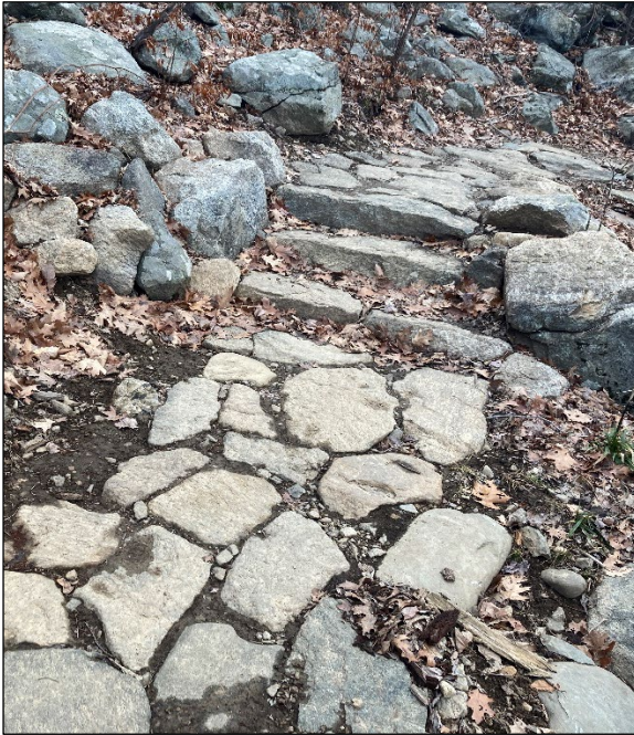
Armored swale with significant outslope.
