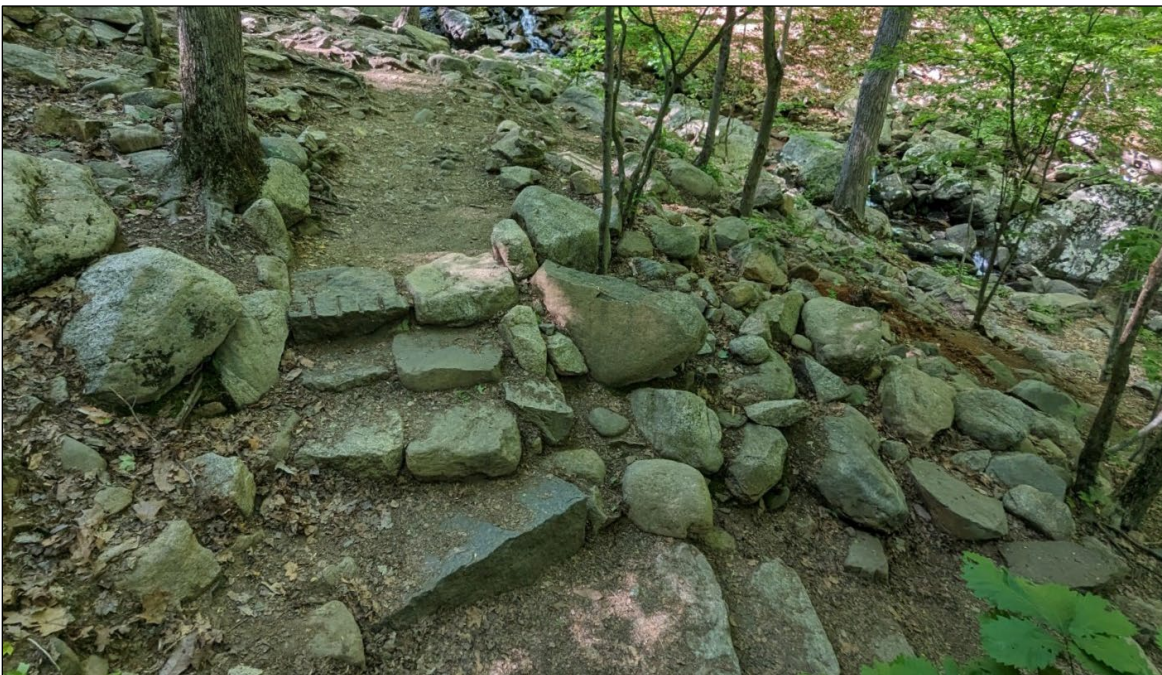
Experienced trail builders can build curved staircases to follow the terrain organically.
