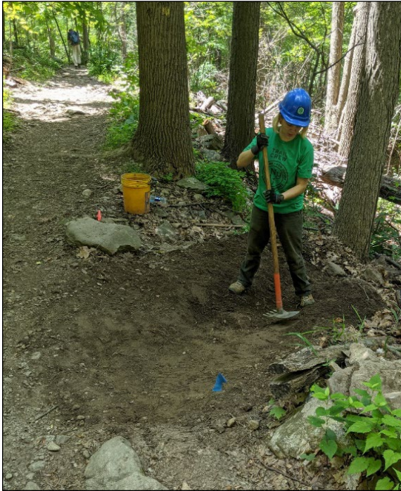
"Punch-Out" Drainage Dip
